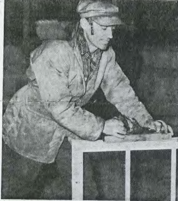
Foreman Trowbridge planes window to fit in new rink building —STAR PHOTO
