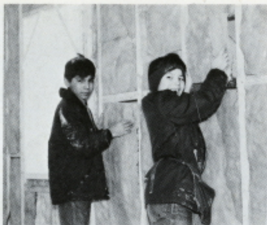
The shop boys put sawdust in the ceiling and fibreglass in the walls and floor to insulate the new house. Ivan
