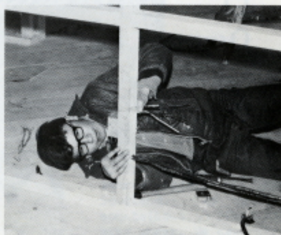
We use 12-2 wires for the receptacles and 14-2 wires for the lights. We staple the wires inside the walls. Ernest
