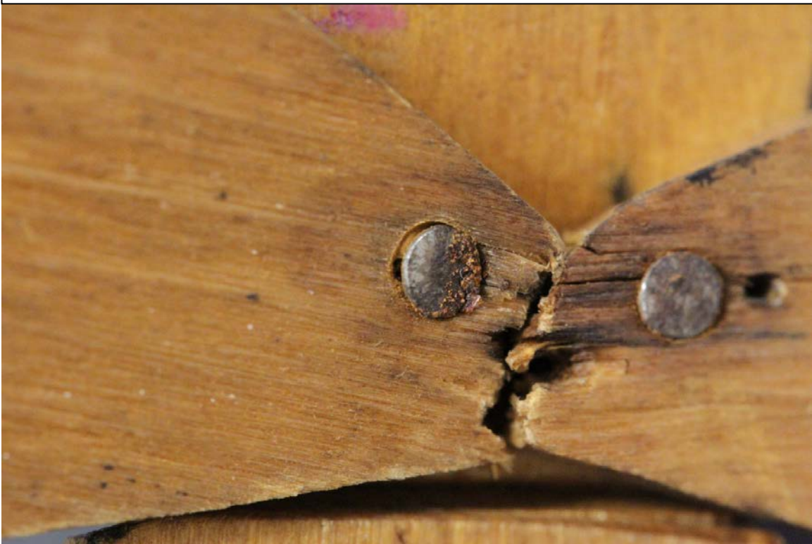
Fig.2 – Corrosion – Back top
