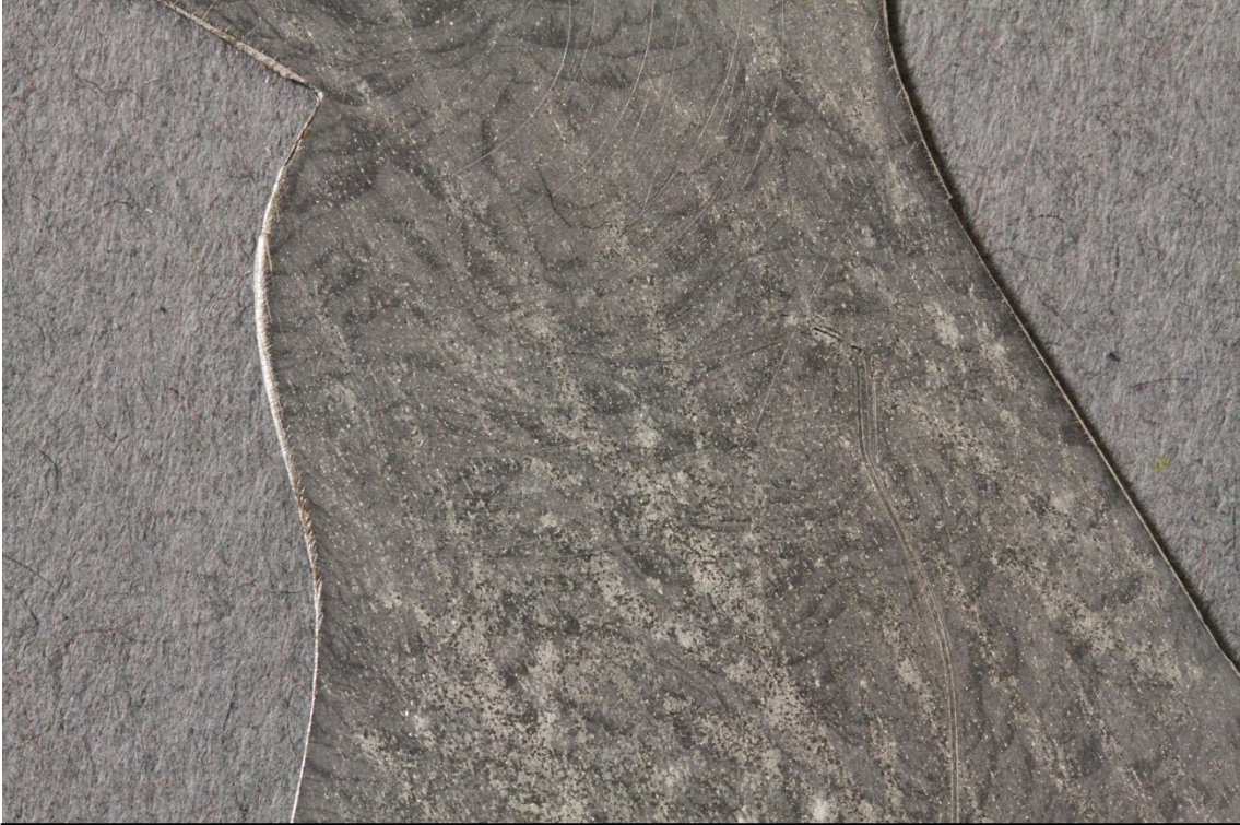
Fig.3 – Corrosion – Back center
