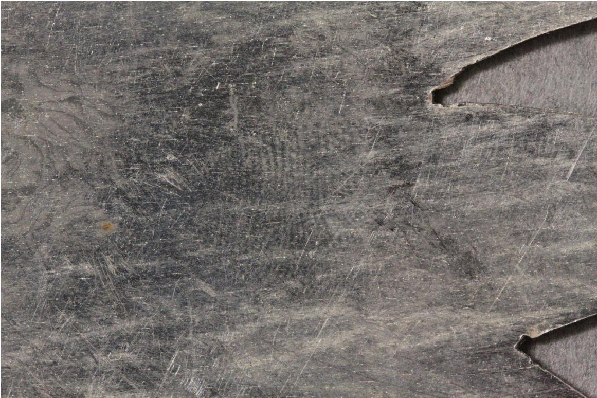
Fig.1 – Corrosion – Front left
