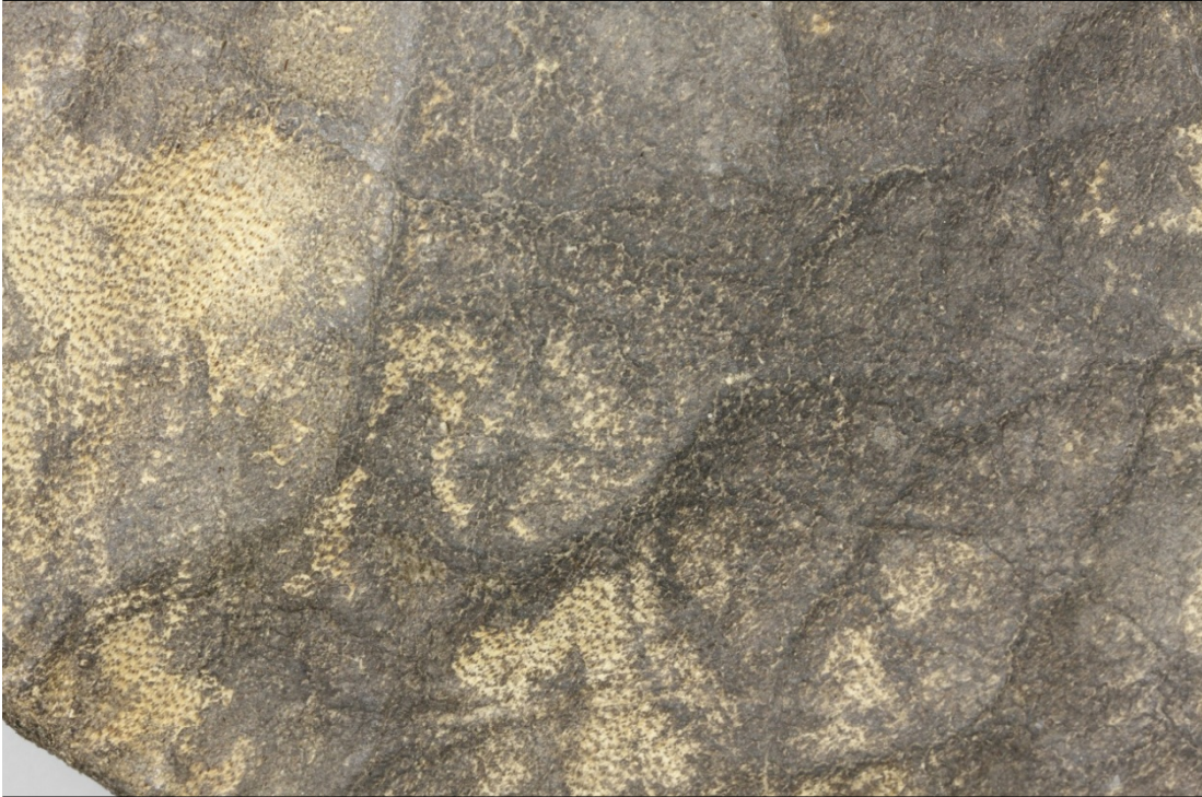
Fig. 8 – Cracking – Bottom front left side
